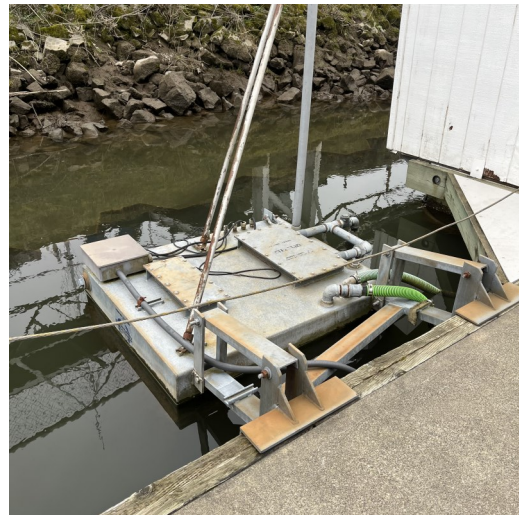
Sewage holding tank and pump station
