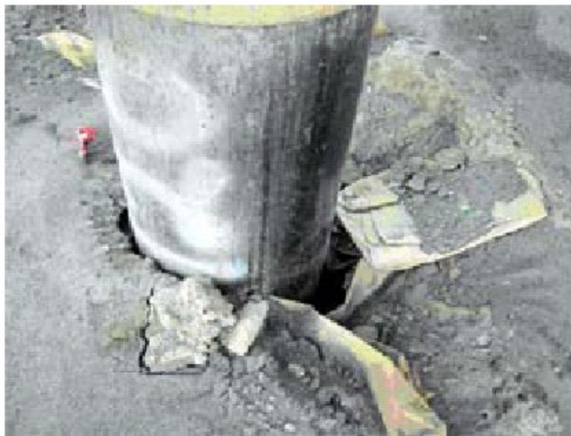
Figure 2. Cement bag seal?
