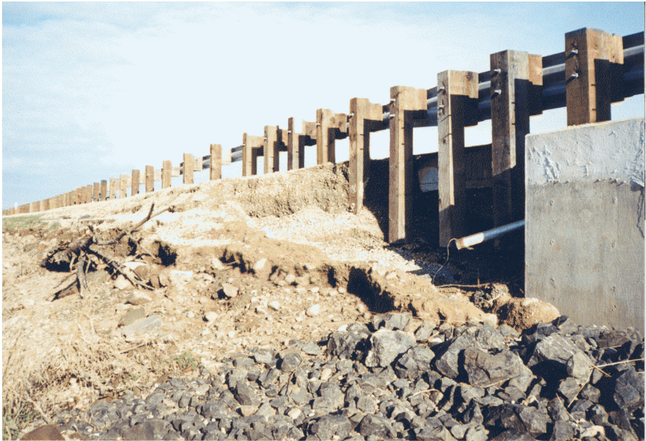
Figure 10-18 Undermined End Panel
