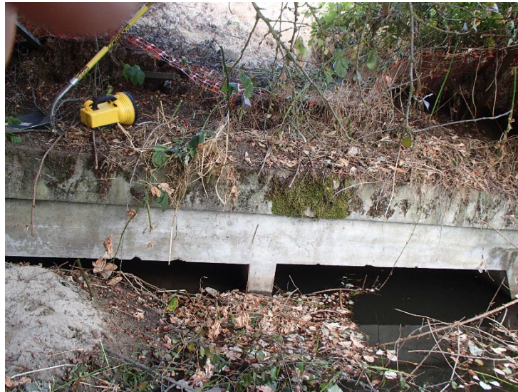
Figure 9 - 3 Inlet sediment accumulation
