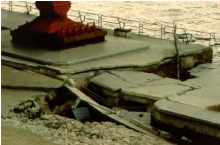
Figure 2.33: Foundation Damage at Kobe Ohashi Bridge
