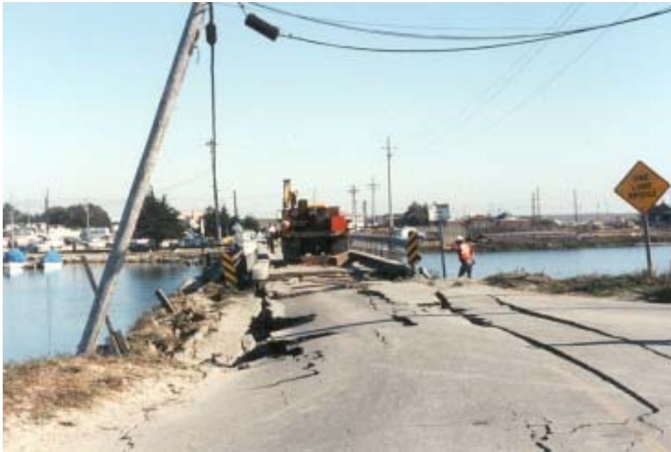
Figure 2.23: Excessive Settlement of Approach Fill
