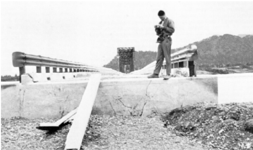
Figure 2.10(b): Post-earthquake Settlement at Copper River Bridge 334
