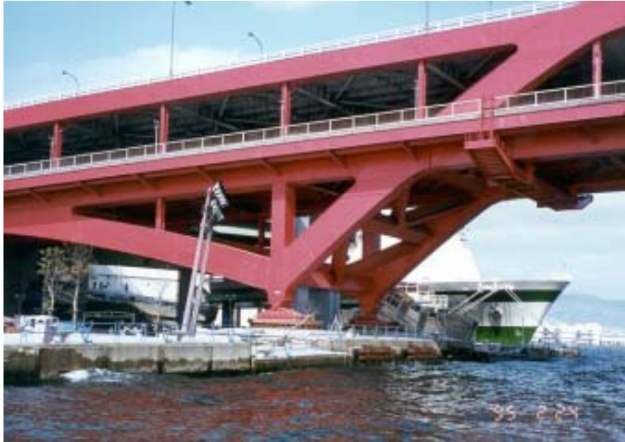
Figure 2.32: Kobe Ohashi Bridge Damage
