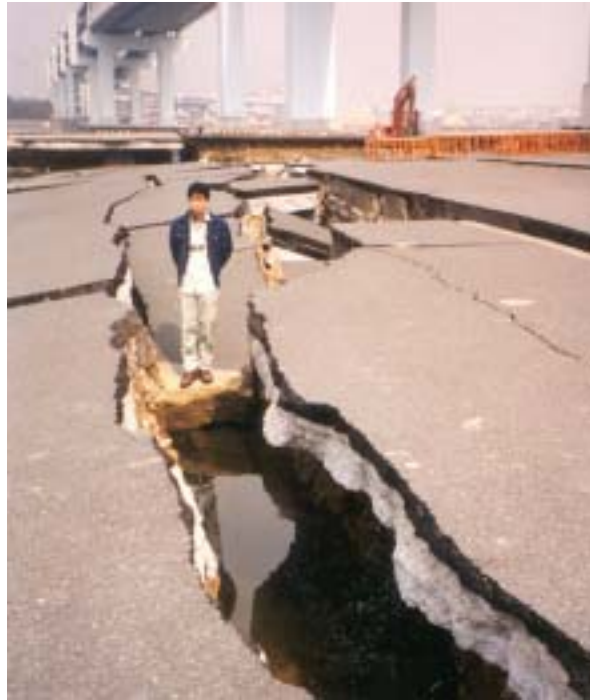
Figure 2.30: Damage to Rokko Ohashi Bridge
