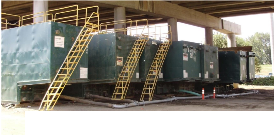
Figure 3-36 Array of Baker Tanks
