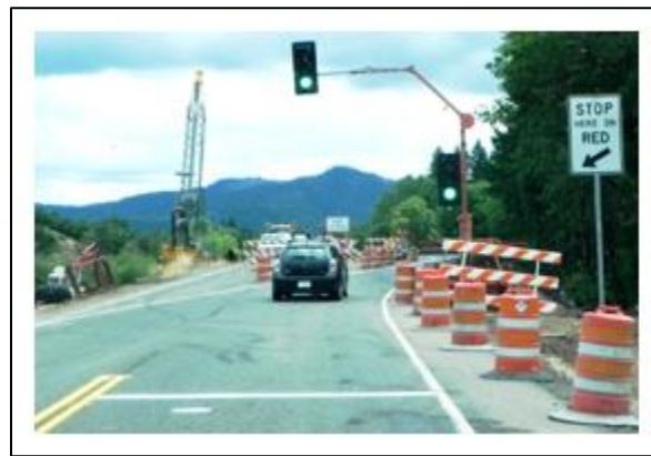
Figure A-1: Portable Traffic Signal
