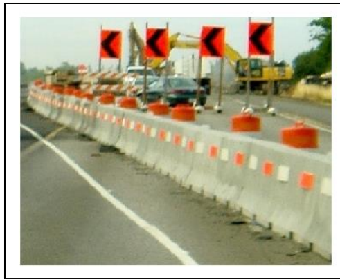
Figure A-1: Reflective Barrier Panels
