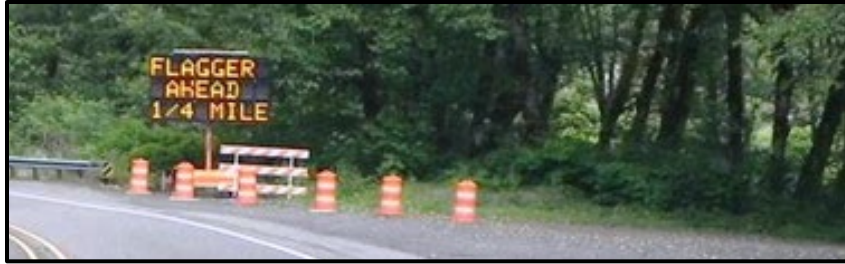
Figure 2 - PCMS located near a pullout for ease of accessibility.
