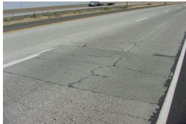
Moderate – patch has moderate longitudinal cracks
