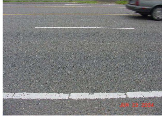
No raveling (open-graded surface)
