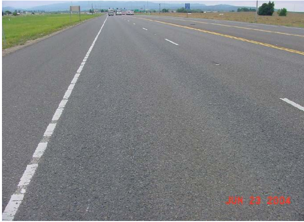
No raveling (open-graded surface)
