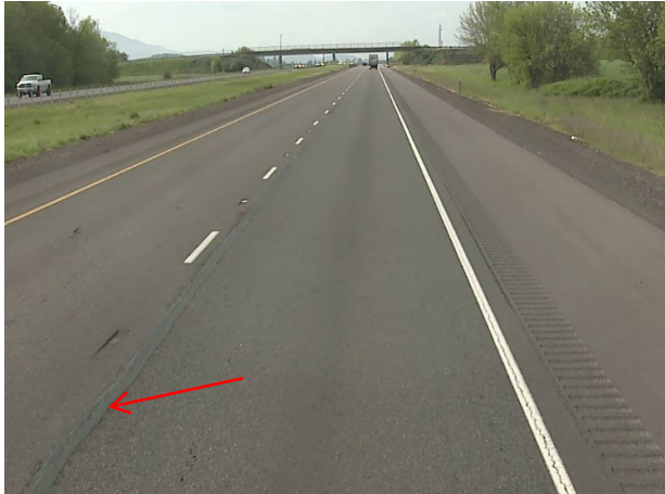
Left edge – sealed severity
