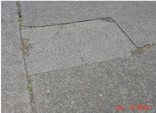
Moderate – patch displays faulting < 0.25"
