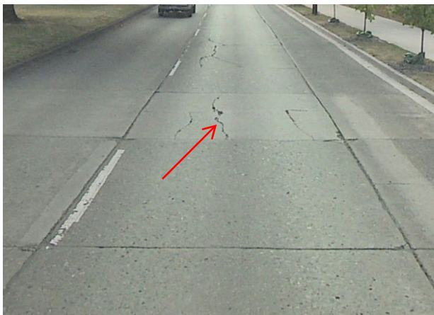
High – patch has high severity distress
