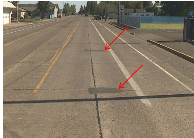
Moderate – small irregular-shaped asphalt concrete patches
