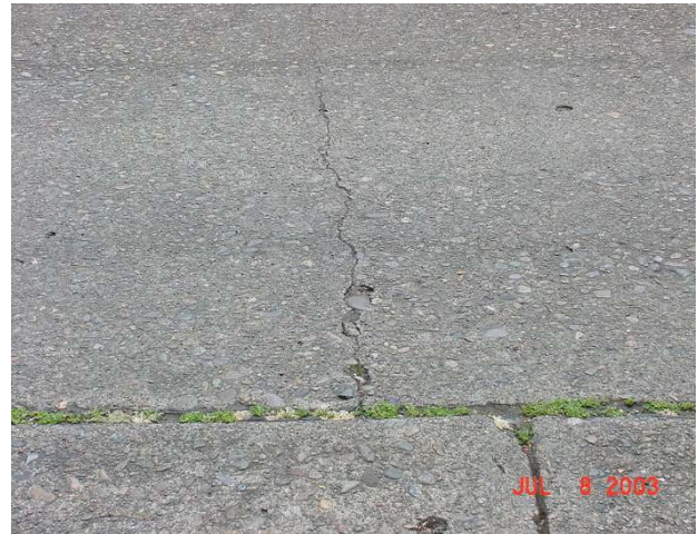
Moderate – transverse crack has spalling
