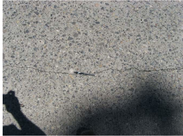
Up close picture of the crack
