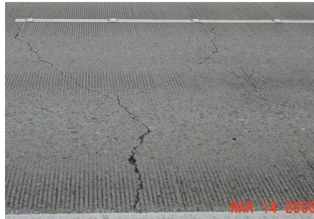
“Y”-crack – do not record as a punchout since branches are not exhibiting spalling, only the trunk is spalling
