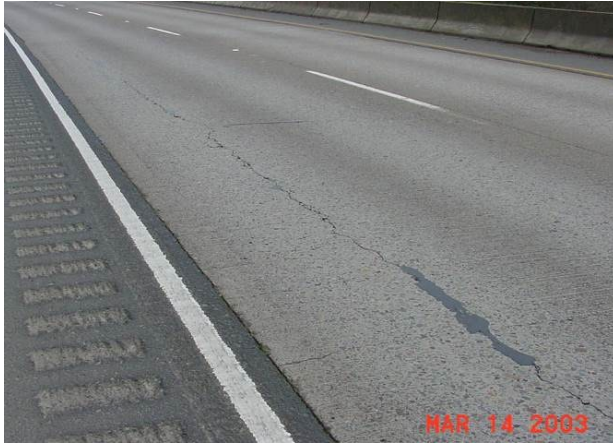
Low – left wheel path (sealed crack)
