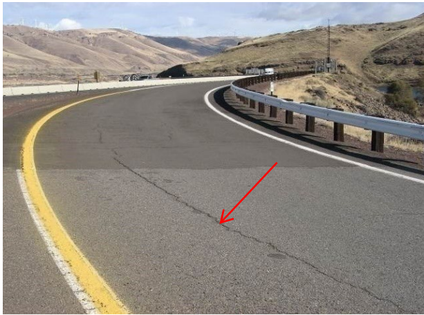
Center – low severity
