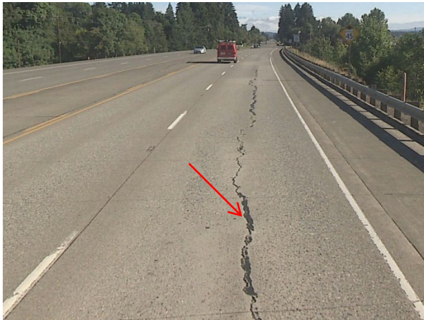
Center – moderate severity (red arrow)
