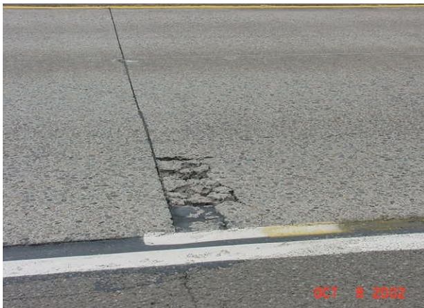
High – faulted over 1/2"
