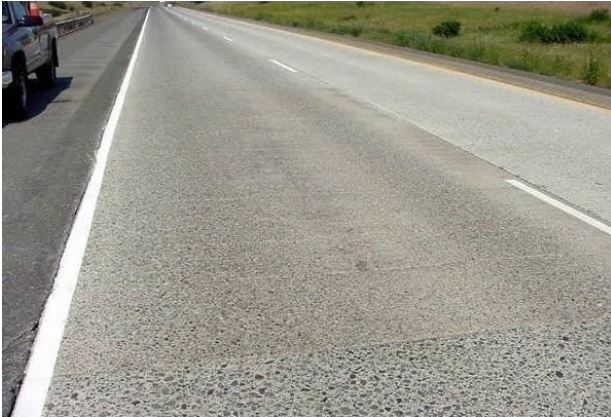
Low severity patch, note tight T-cracks
