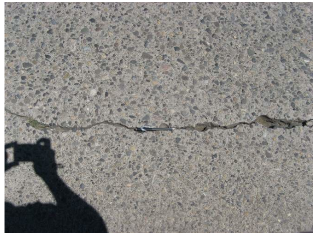
Up close picture of the crack
