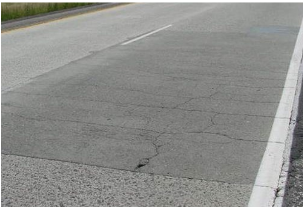
Moderate – patch has longitudinal crack with spalling
