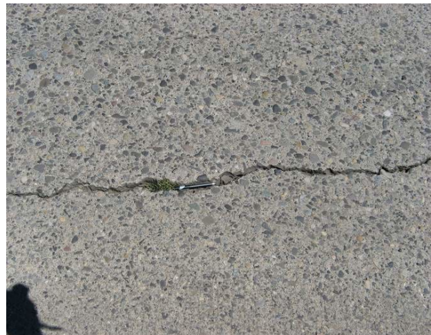
Up close picture of the crack
