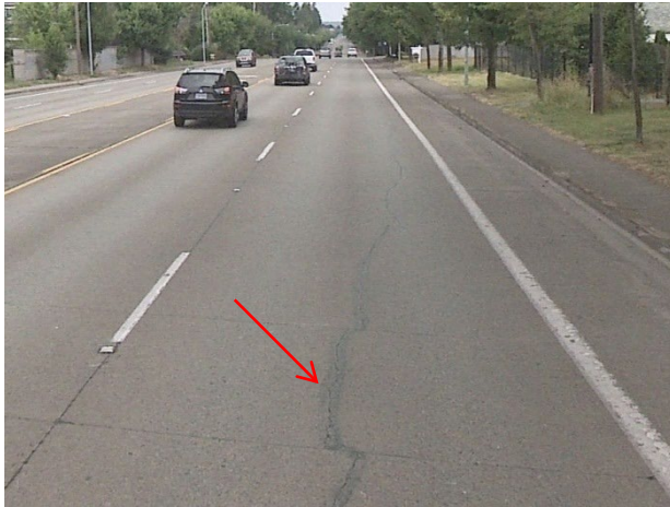
Center – low severity (red arrow)
