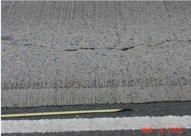
Not a punchout, spalling on L-crack only
