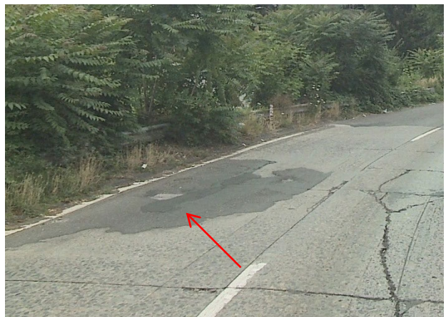
High – patch is severely deteriorated
