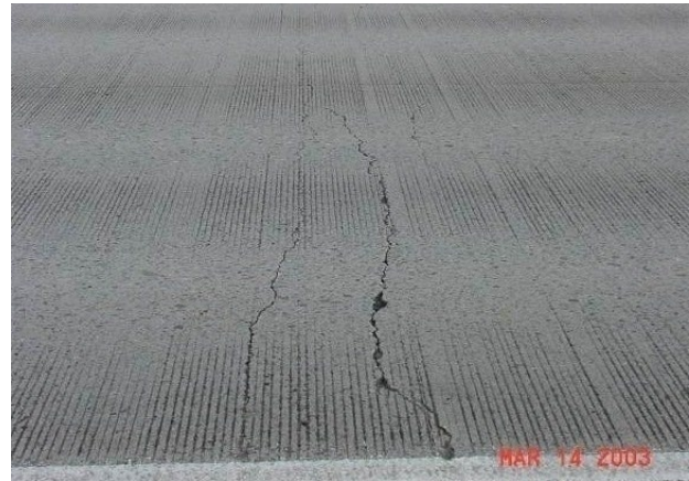
Not a “Y”-crack based on the 1/2 lane rule
