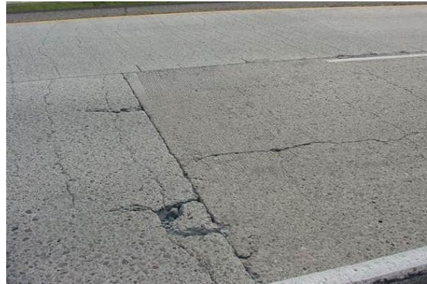
Moderate – spalling between 3” and 6”
