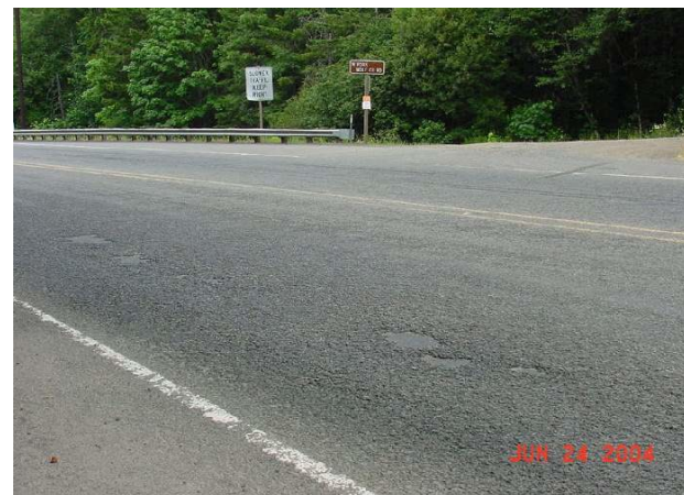
High (with potholes)
