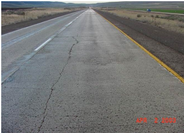
Moderate – left wheel path (due to spalling)
