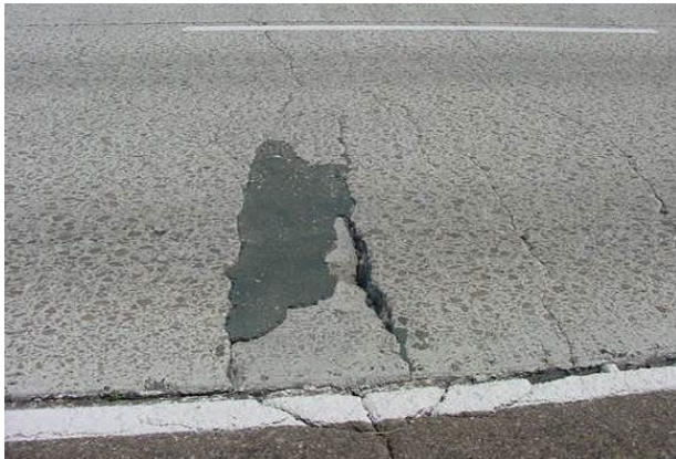
High – more than 0.5” faulting
