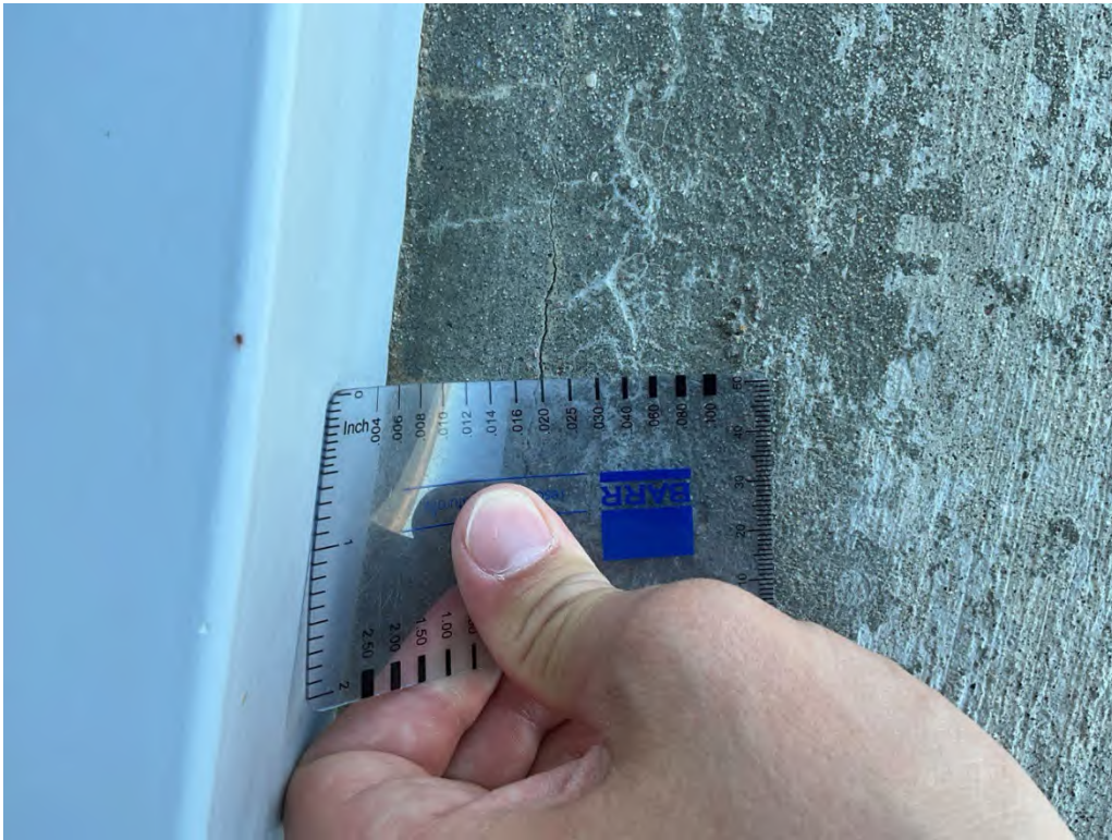
Figure 3-4 Example of grout circumferential cracking
