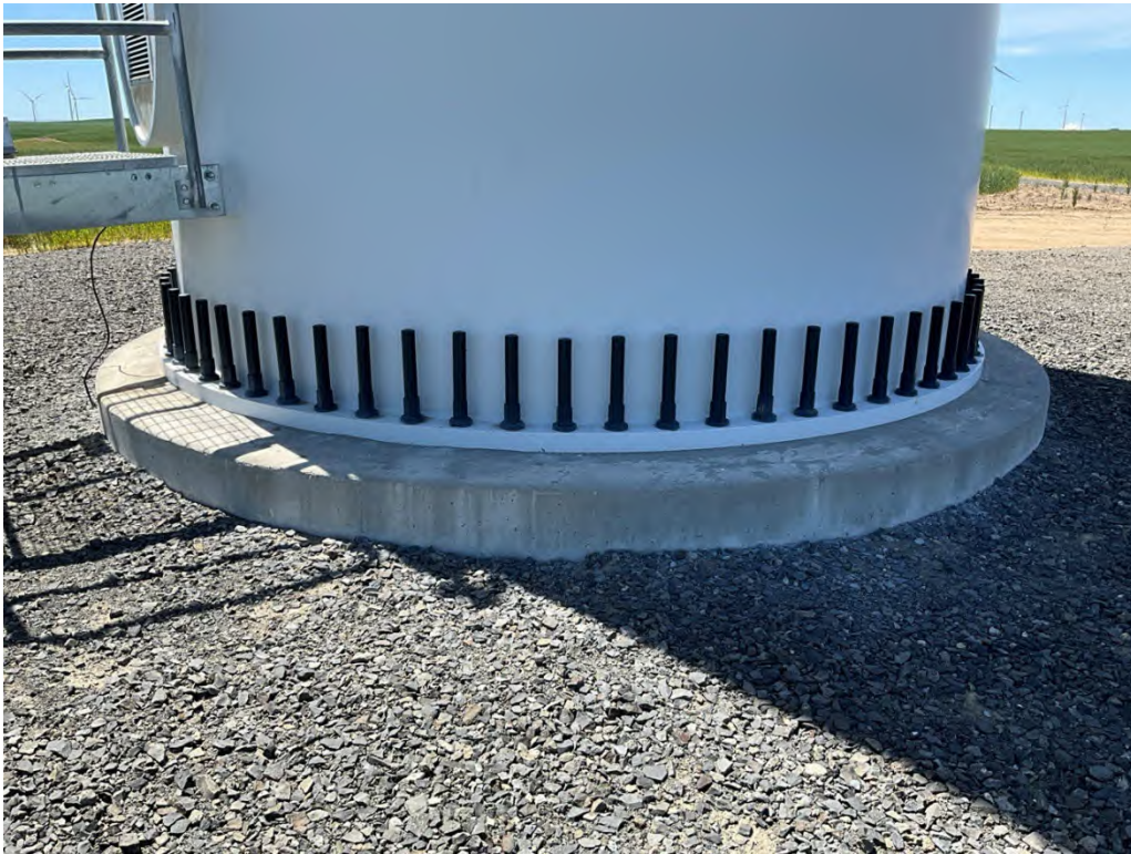
Figure 3-2 Example of low backfill condition
