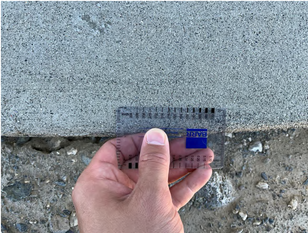
Figure 3-6 Example of pedestal radial cracking
