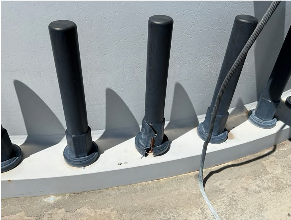
Figure 3-8 Example of damaged/missing anchor bolt covers
